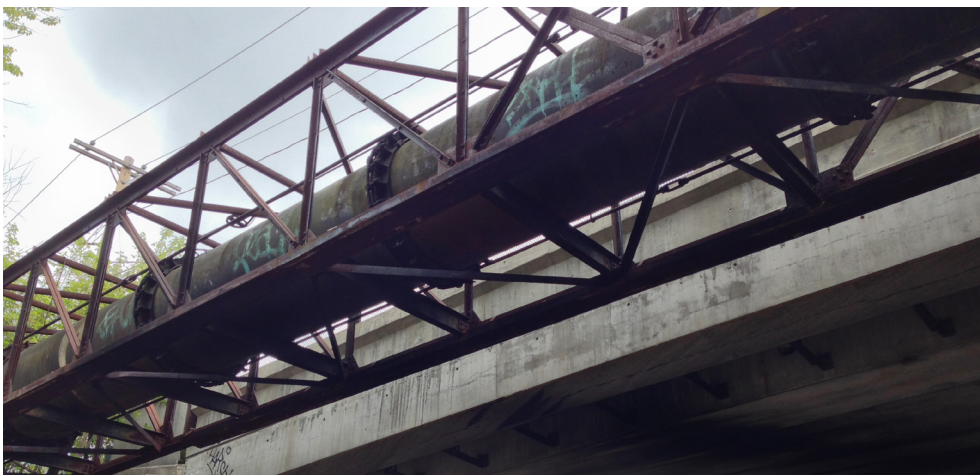
Figure A5.2.9-2: Walnut Street Bridge utility bridge with 48-in. MWRA water main. By bringing the Community Path to street grade, GLP reduces the cost and risk of tunneling under this vital pipeline
