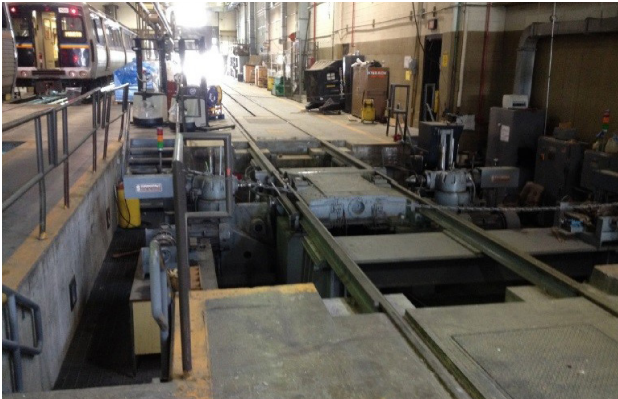
Figure A5.2.5-8: GLP's design relocates the wheel true pit to an exterior wall to isolate wheel truing from other maintenance functions. This design has the benefits of improved shop circulation and ease of maintenance.
