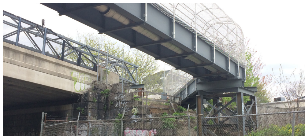
Figure A5.2.9-4: School Street roadway and utility bridges. After GLP constructs the new span for the roadway bridge, the water main will be relocated back to the roadway bridge and the temporary utility bridge will be removed, providing additional space in the ROW for other Project elements.
