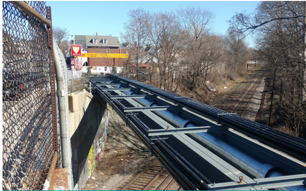
Figure A5.2.9-6: GLP will convert the temporary utility bridge at Broadway into a permanent structure, thereby reducing the cost and service interruptions to customers associated with relocating utilities back to the roadway bridge
