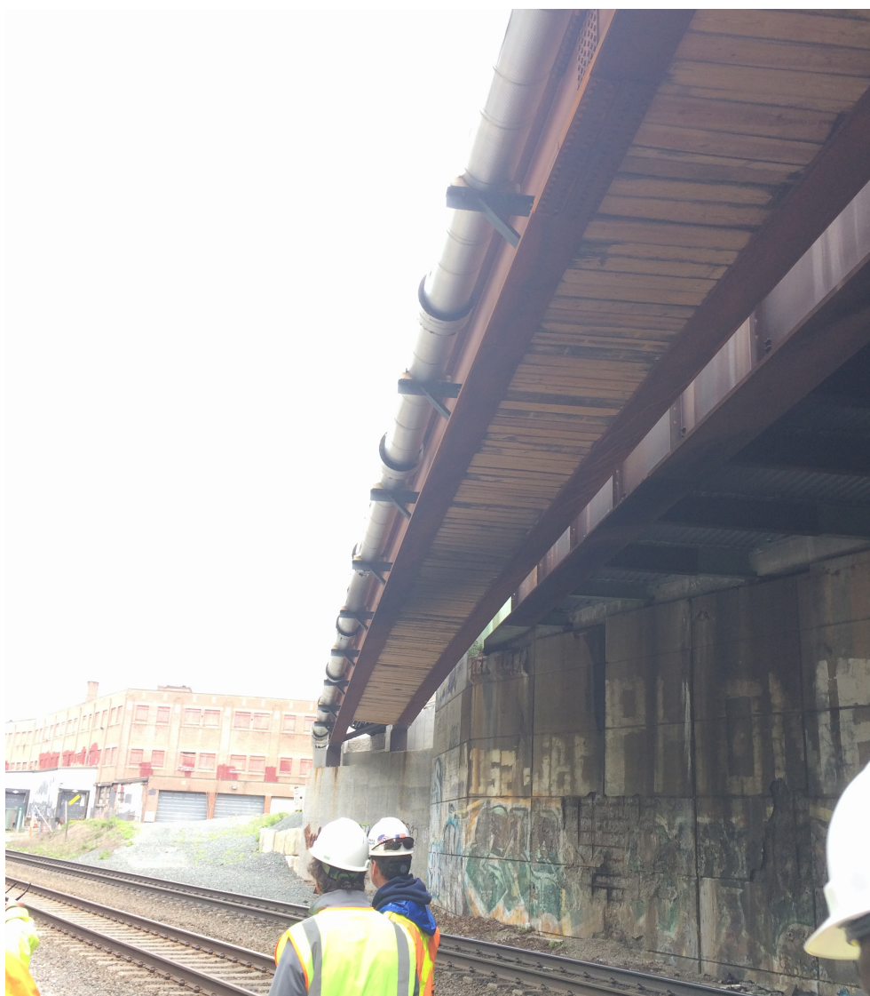
Figure A5.2.9-3: GLP will convert the temporary utility bridge at Medford Street into a permanent structure, thereby reducing the cost of relocating utilities back to the roadway bridge
