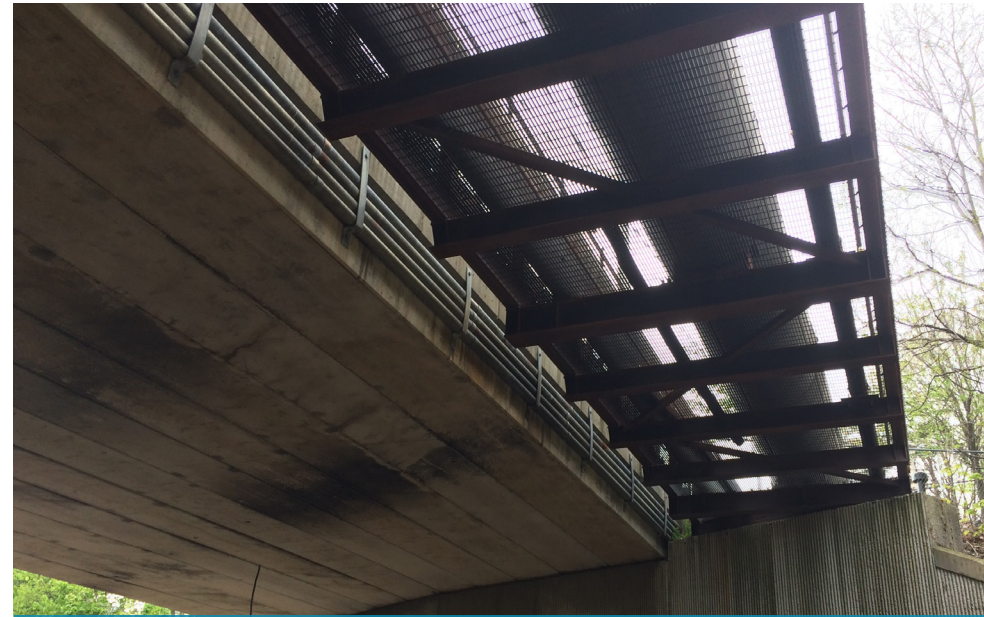
Figure A5.2.9-7: GLP will convert the temporary utility bridge at Broadway into a permanent structure, thereby reducing the cost and service interruptions to customers associated with relocating utilities back to the roadway bridge.
