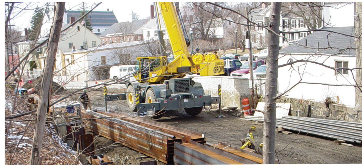
Figure 4.9-1. The Construction of the Hingham Tunnel required coordination and relocation of numerous utilities including the 54" Town Brook Culvert. The project was successfully completed on time.
