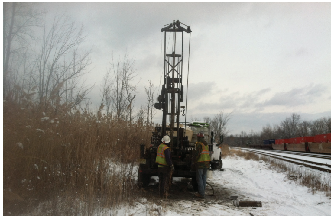
Field engineers overseeing subcontractors drilling environmental borings and taking soil samples along a railroad Right of Way.
