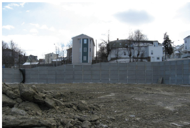
Figure 4.2-14. Drilling Soldier Pile and Permanent Precast Concrete Lagging wall. Used for wall heights up to 28 feet without impacting adjacent structures.
