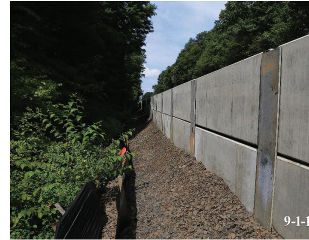
Figure 4.2-8. Soldier Pile and Precast Concrete Lagging Wall Construction. Use where open-cut excavation is precluded and to limit ground movement adjacent to existing structures.
