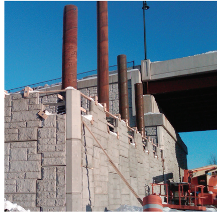
Figure 4.2-6. Viaduct Foundations at MSE wall interface. Viaduct foundations will not bear on the MSE embankments.
