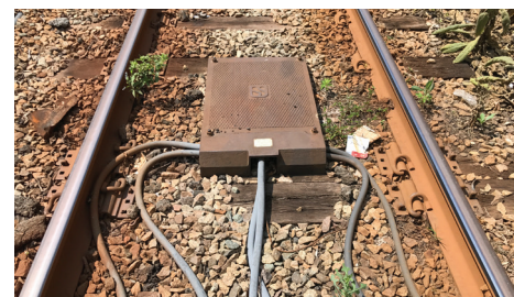
Impedance Bond (IB). The following is an example of an IB which may be used on the Project.
