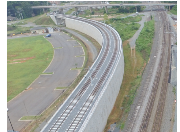
Light rail track supported by Mechanically Stabilized Earth (MSE) walls. GLX Constructors' team members, Balfour Beatty and STV, incorporated the use of low maintenance MSE walls on the Charlotte LYNX Blue Line Light Rail Project in North Carolina.
