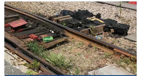
Switch Machine. The following is an example which may be used on the Project.
