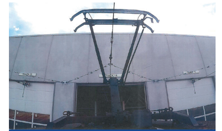
MBTA Orient Heights Blue Line Car House. A similar door system will be used at the VMF to accommodate the OCS.
