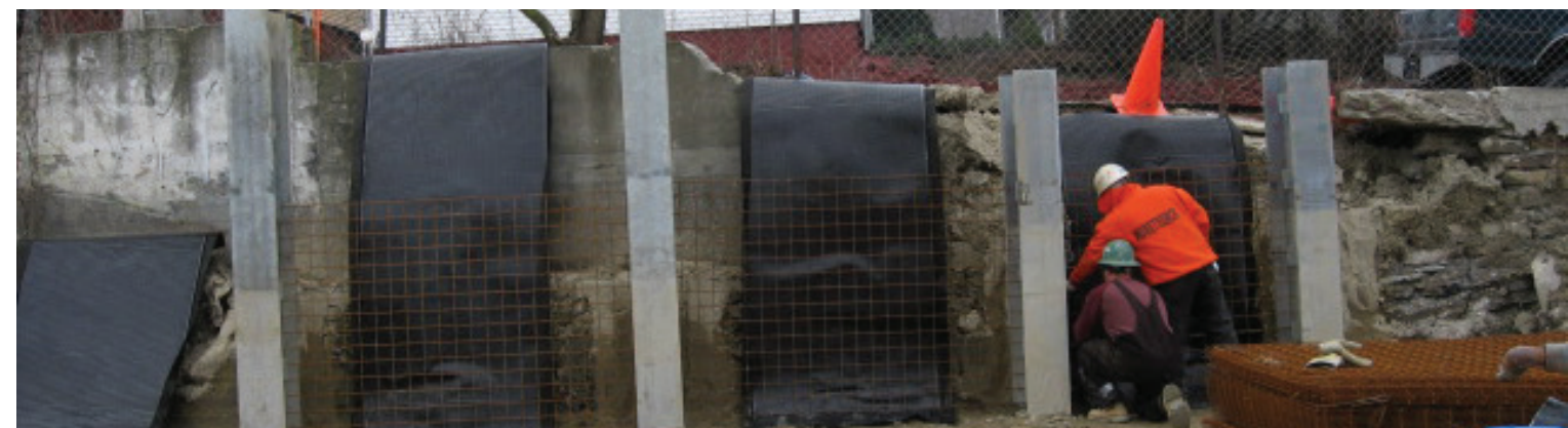
Figure 4.2-11. Installation of Drainage Board behind Shotcrete Walls. Where shotcrete is used, the boards will assure effective drainage behind the completed wall system.
