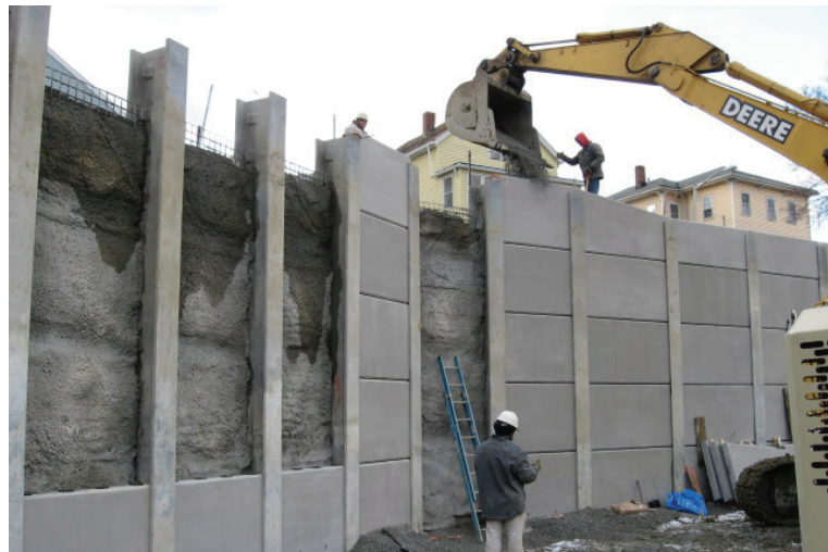
Figure 4.2-12. Precast concrete panels and drilled soldier piles. GLX Constructors have experience with designing and installing drilled soldier pile and permanent precast concrete lagging walls using shotcrete as temporary support.
