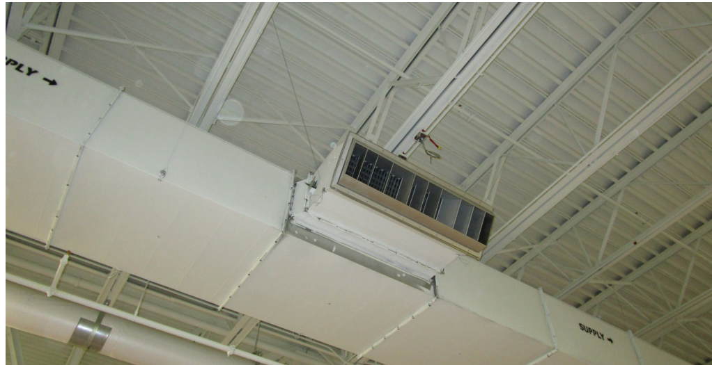
Figure 4.5-2. Roof-Mounted Air Handling Unit. Example.
