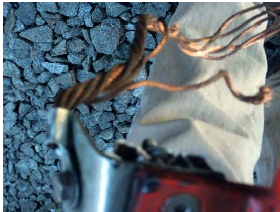
Figure 6.6.2-4 Power Asset Deficiency: Frayed Conductor
