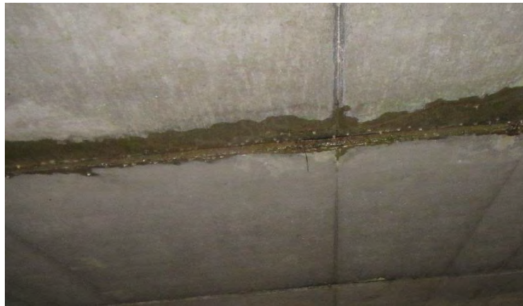
Figure 6.2.1-8 Concrete Deficiency: Differential Settlement
