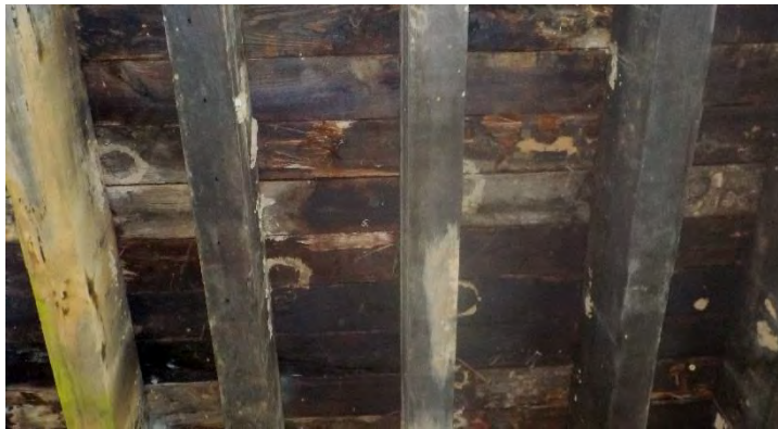
Figure 6.2.4-1 Timber Deficiency: Decay or Rot
