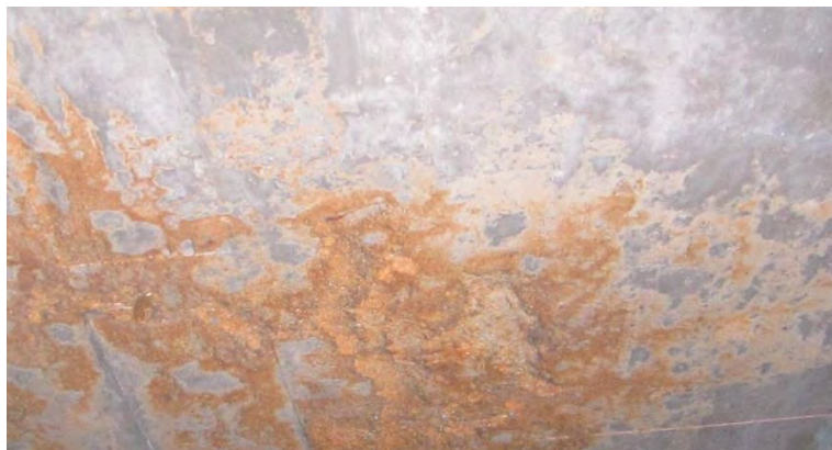
Figure 6.2.1-4 Concrete Deficiency: Rust Staining
