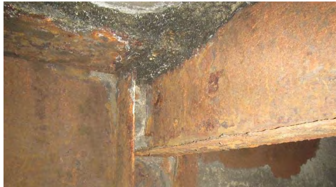
Figure 6.2.2-2 Steel Deficiency: Moderate Corrosion
