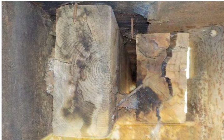
Figure 6.2.4-2 Timber Deficiency: Cracks and Splits
