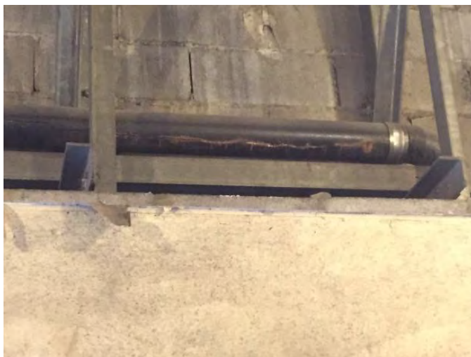
Figure 6.3.1-1 Drain System Deficiency: Cracked Pipe
