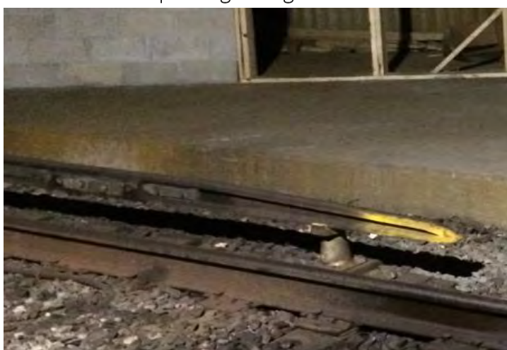
Figure 6.6.3-10 Track Asset Deficiency: Cable
