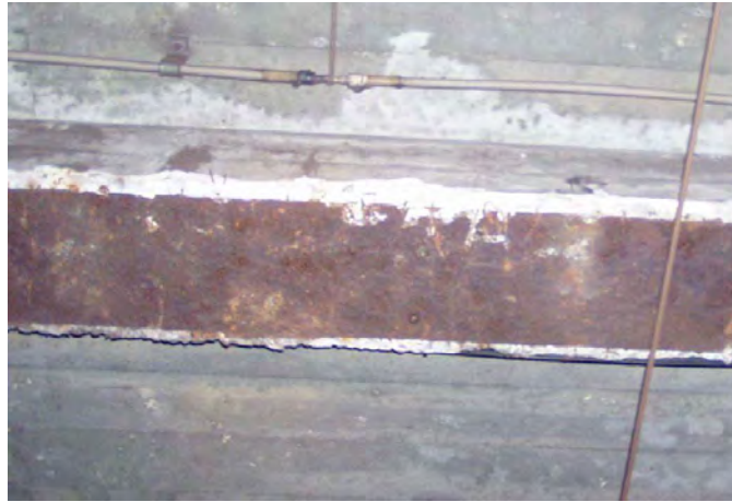
Figure 6.2.2-1 Steel Deficiency: Light Corrosion
