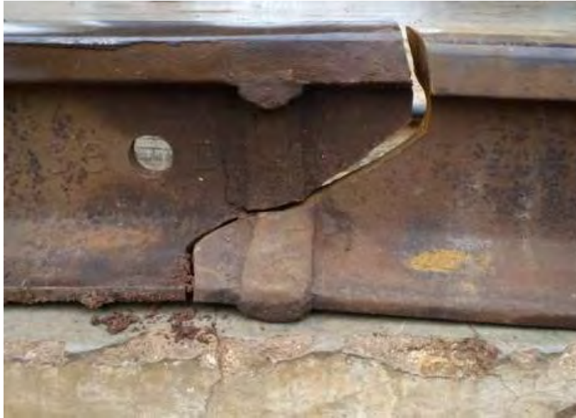
Figure 6.6.3-2 Track Asset Deficiency: Weld Failure
