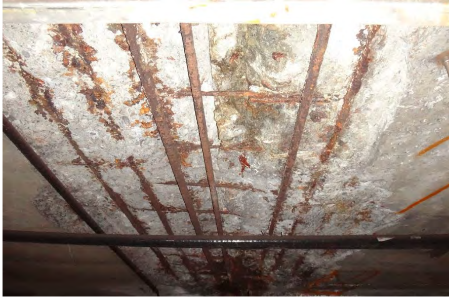
Figure 6.2.1-1 Concrete Deficiency: Spall with Exposed Reinforcing Steel
