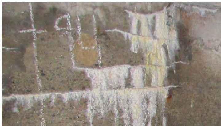
Figure 6.2.1-5 Concrete Deficiency: Efflorescence
