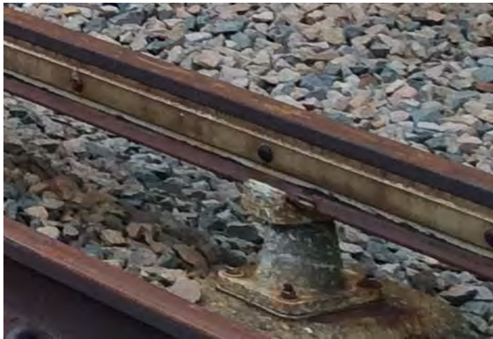
Figure 6.6.3-7 Track Asset Deficiency: Cable
