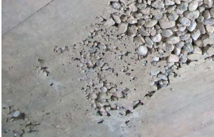
Figure 6.2.1-7 Concrete Deficiency: Honeycomb
