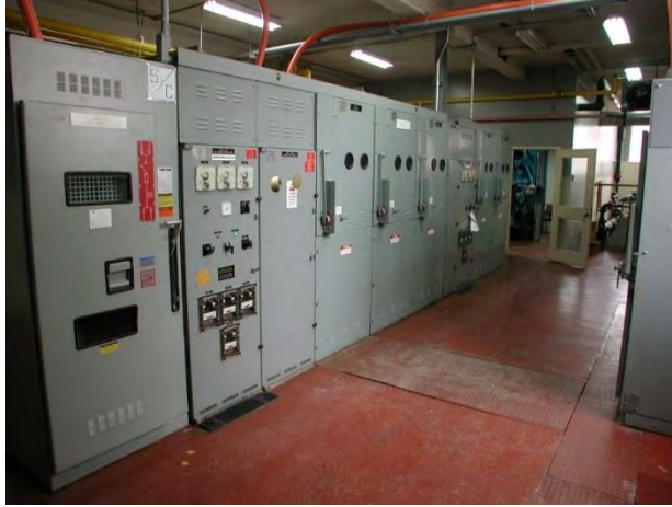
Figure 6.6.2-6 Typical Electrical Room
