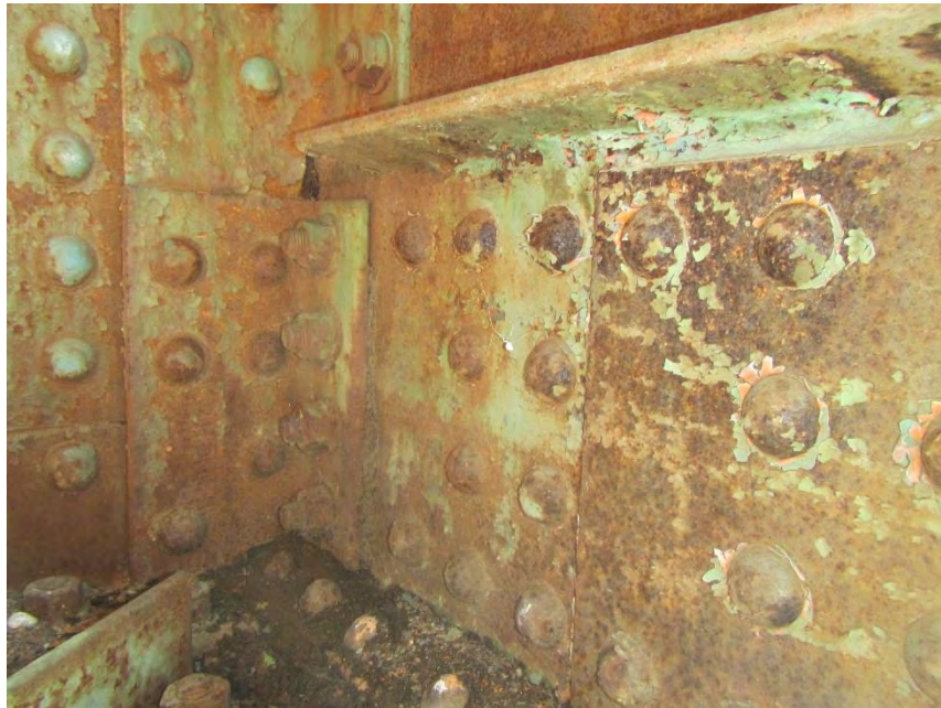
Figure 6.2.2-4 Steel Deficiency: Connection (Light Corrosion)
