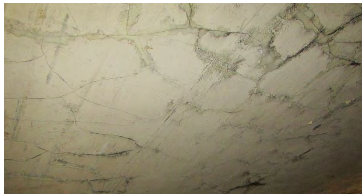
Figure 6.2.1-3 Concrete Deficiency: Map Cracks
