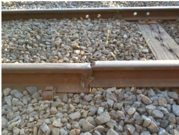
Figure 6.6.3-1 Track Asset Deficiency: Broken Rail
