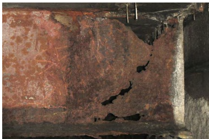
Figure 6.2.2-3 Steel Deficiency: Severe Corrosion
