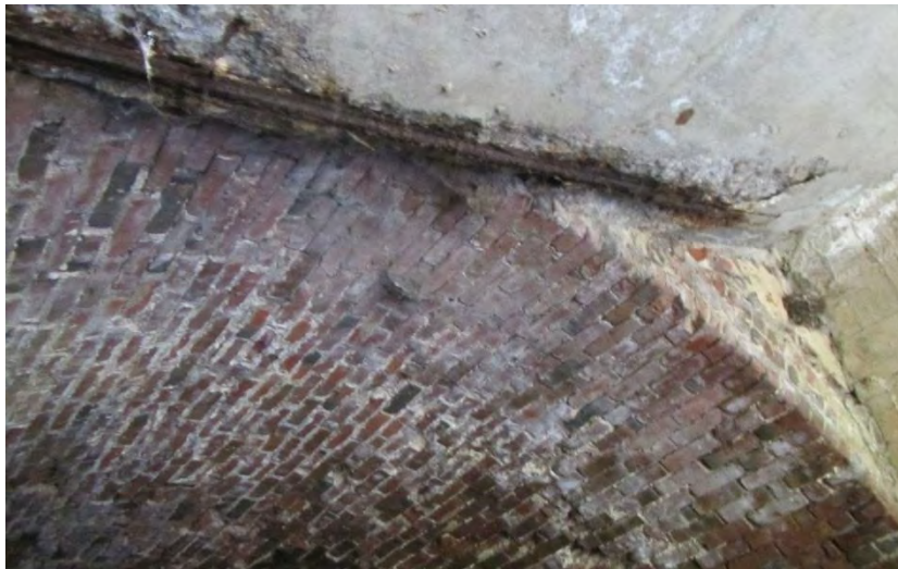
Figure 6.2.3-1 Masonry Deficiency: Mortar Breakdown and Efflorescence
