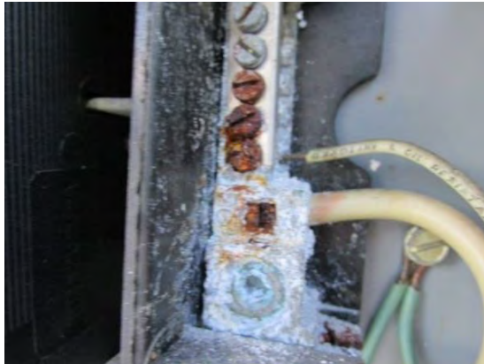
Figure 6.6.2-3 Power Asset Deficiency: Corrosion
