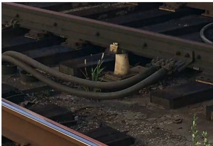
Figure 6.6.3-8 Track Asset Deficiency: Cable
