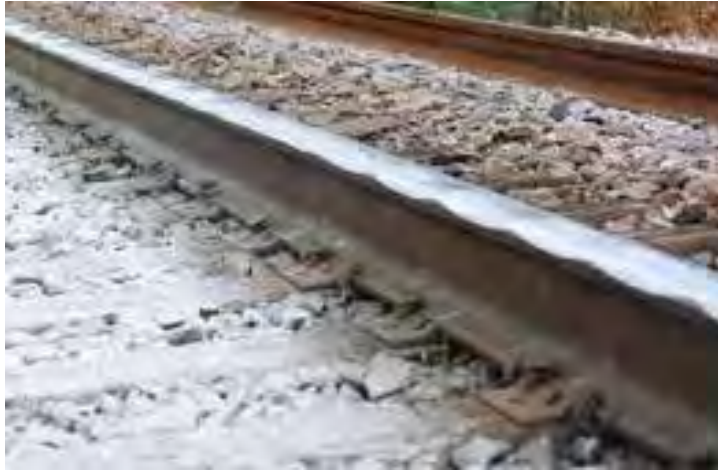
Figure 6.6.3-5 Track Asset Deficiency: Corrugation
