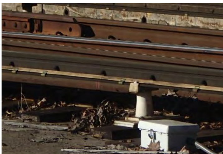
Figure 6.6.3-9 Track Asset Deficiency: Cable
