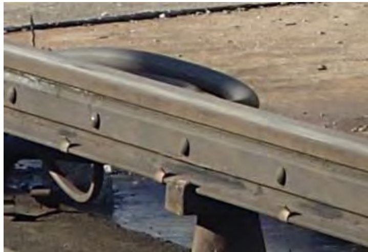
Figure 6.6.3-11 Track Asset Deficiency: Cable
