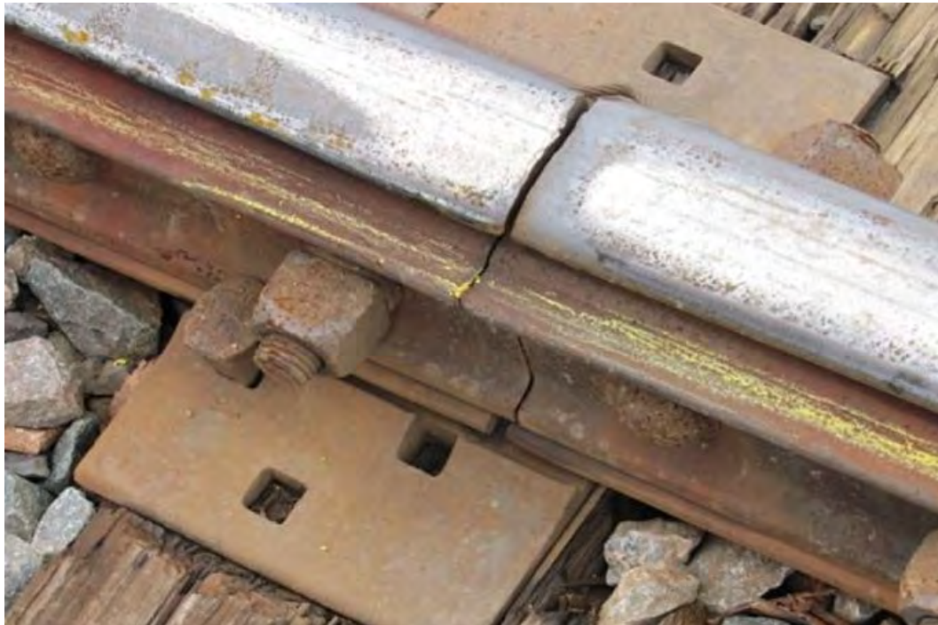
Figure 6.6.3-6 Track Asset Deficiency: Joint Defect
