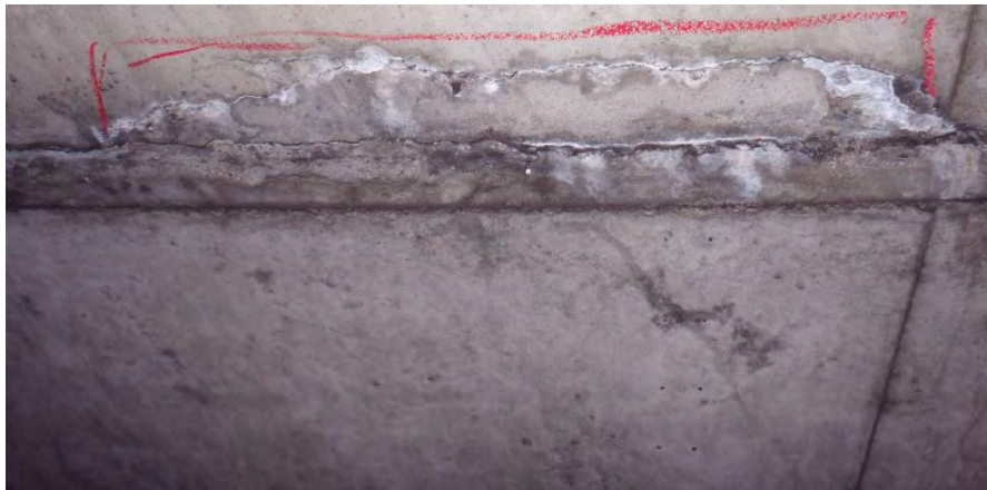
Figure 6.2.1-2 Concrete Deficiency: Delamination
