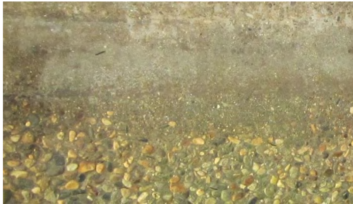
Figure 6.2.1-6 Concrete Deficiency: Scaling
