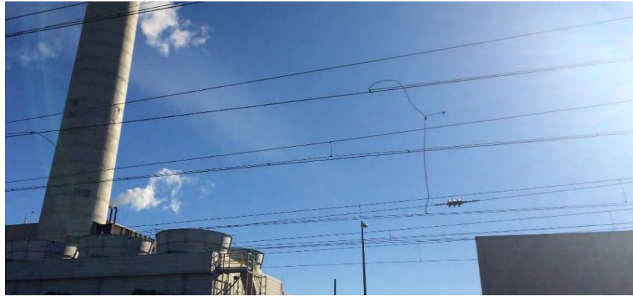
Figure 6.6.2-1 Power Asset Deficiency: Fatigue Break of a Conductor
