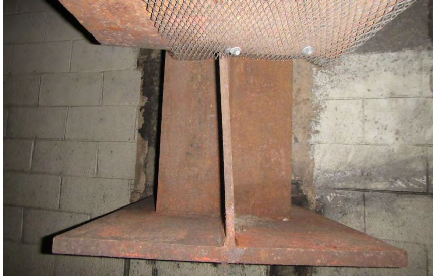
Figure 6.2.2-5 Steel Deficiency: Distortion
