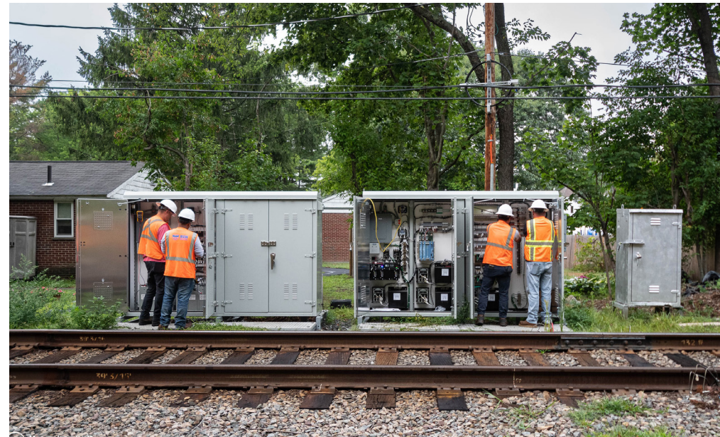
Crew performing work related to PTC/ATC implementation at Commuter Rail signal houses on the Newburyport/Rockport Line.
