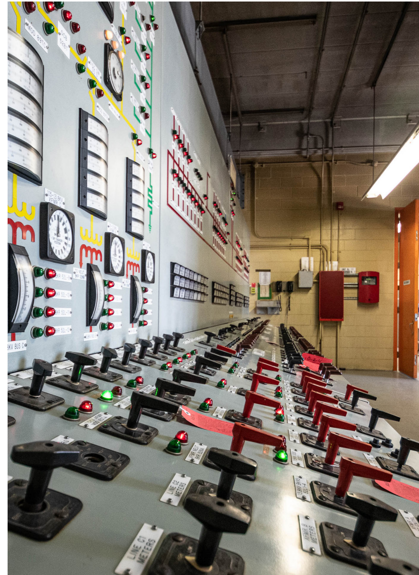
Equipment at the South Boston Switching Station.
