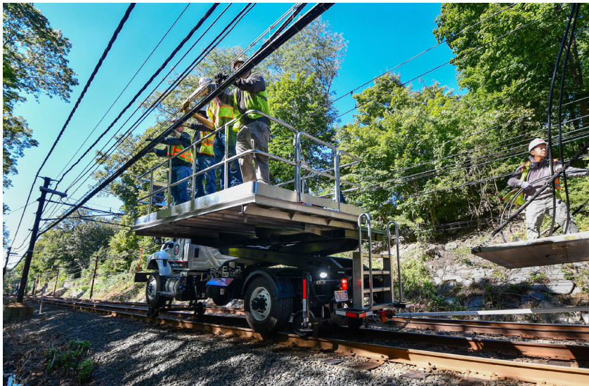
Cable and signal work replacement on the Green Line D Branch near Chestnut Hill station.
