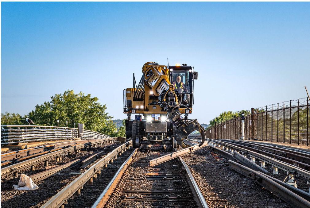
Orange Line rail construction on the Dana Bridge, which carries trains over the Mystic River.
