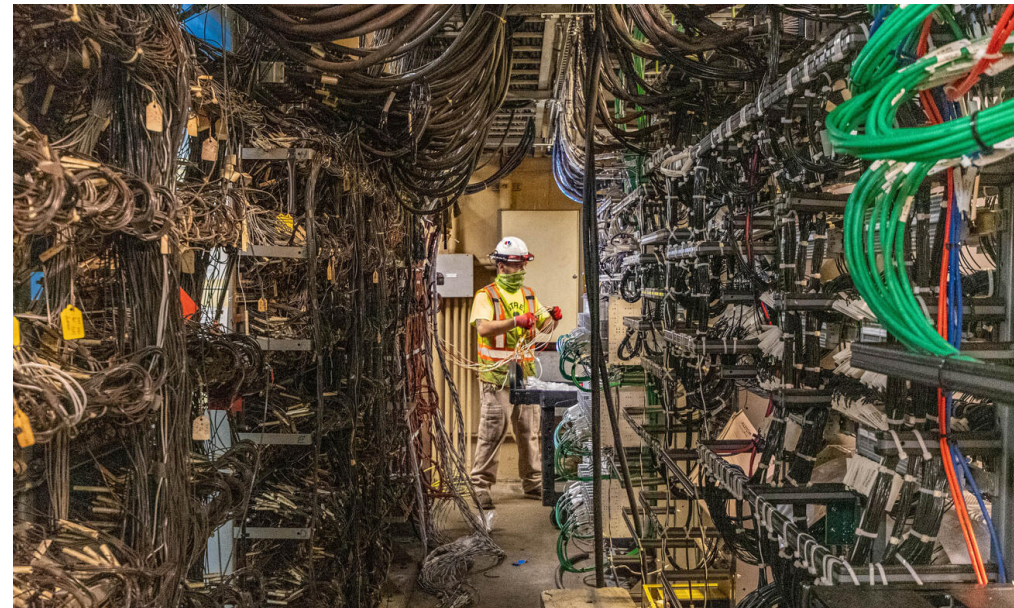
Wire racks in a Red Line signal room.
