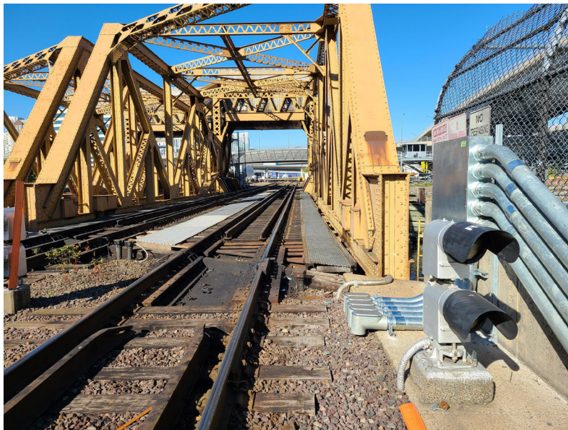
Wayside signal equipment at the North Station Drawbridge.
