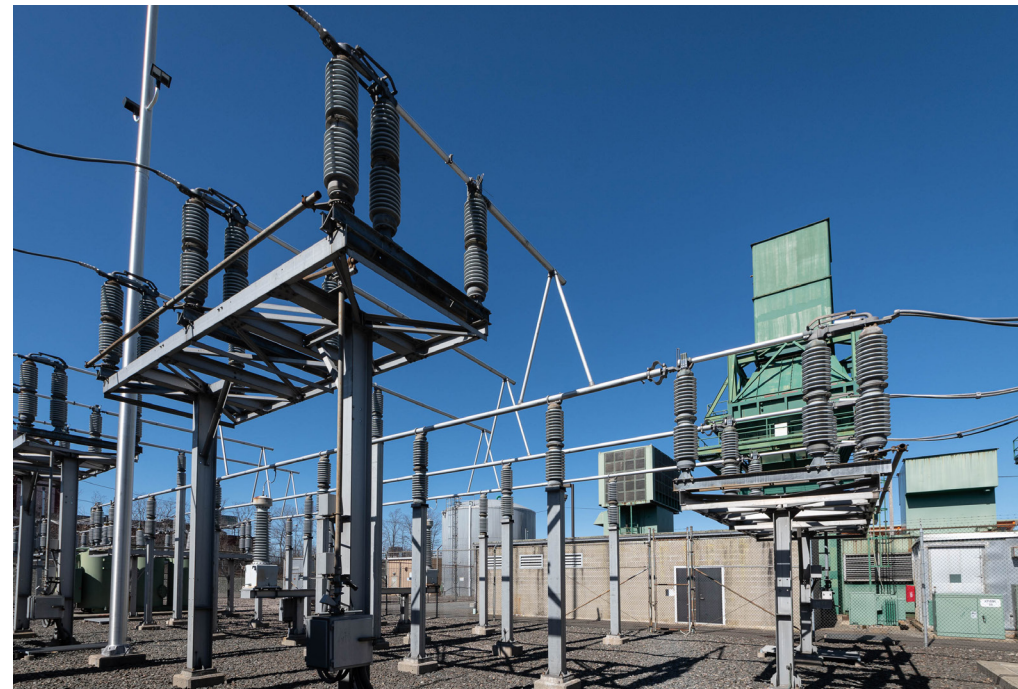
High voltage yard at the South Boston Switching Station.
