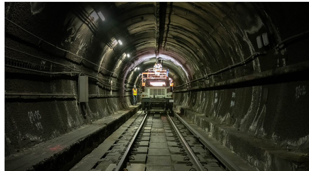
Maintenance work being performed in the Red Line tunnel near Porter Square.
