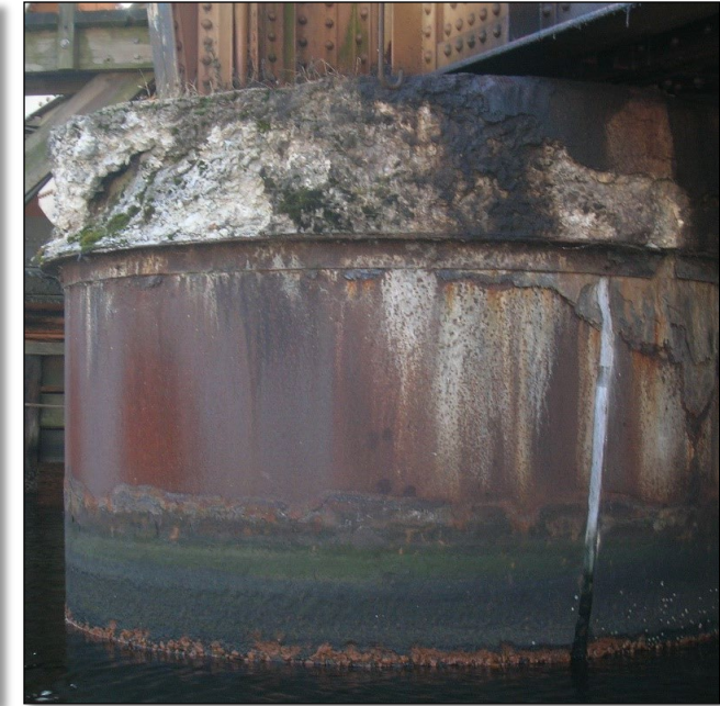
Picture of Bridge Caisson showing deterioration
