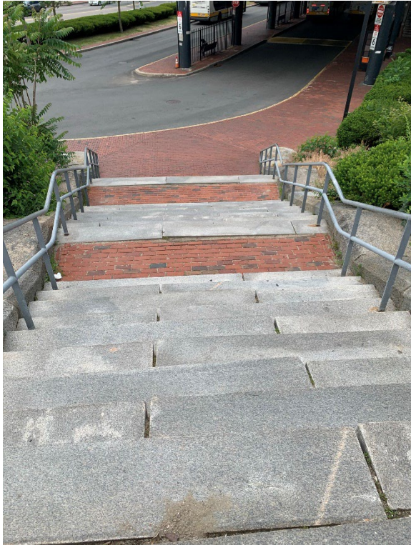
Uneven steps that do not meet ADA standards
