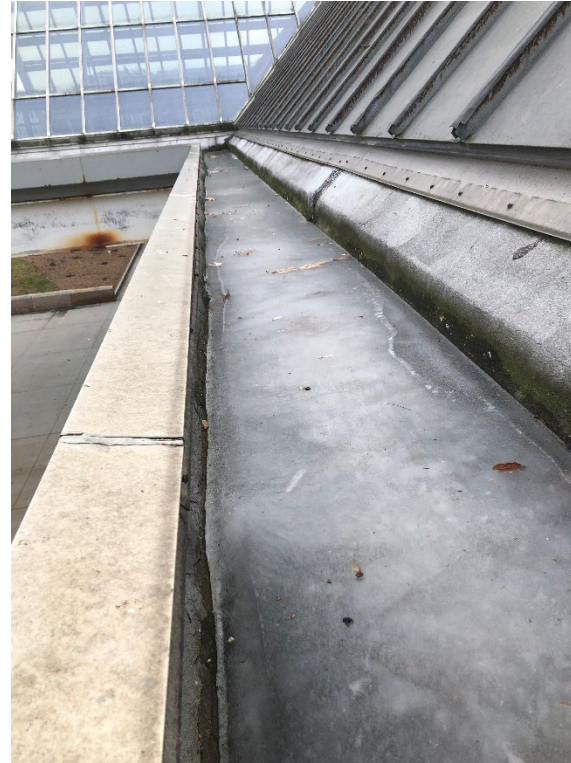
Deteriorated drainage structures
