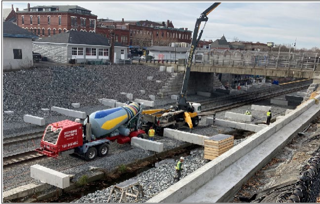
As seen above, construction crew making final placement of the new retaining wall.
