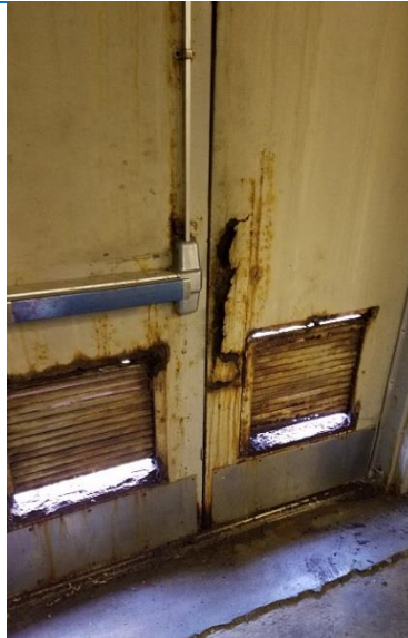
Generator Room Exterior Door, Suffolk Downs Station
