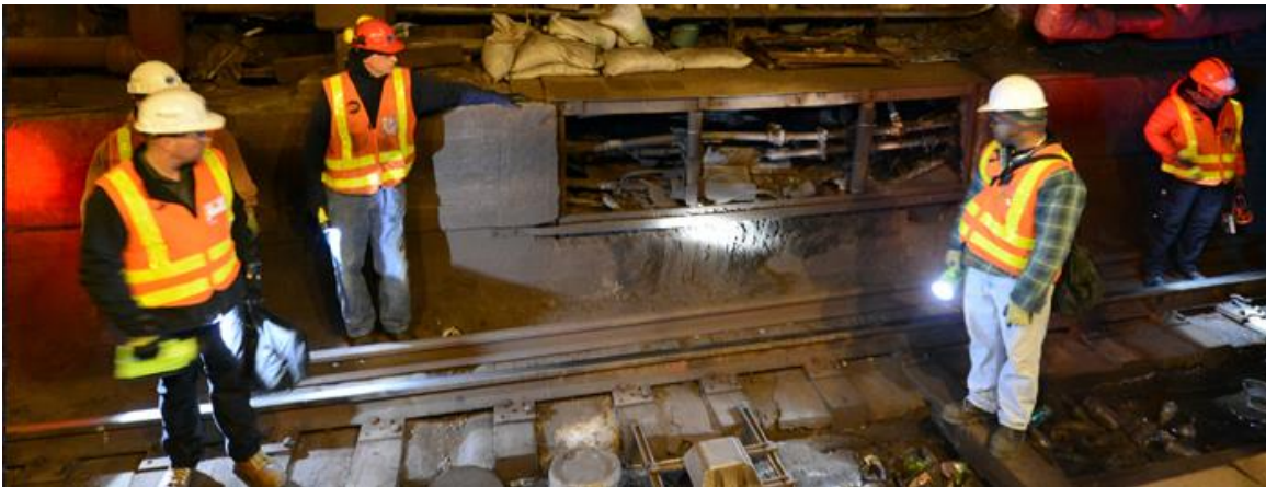
Exhibit 12. Corrosion in New York’s Canarsie Tunnel after Flooding from Superstorm Sandy (Source: MTA 2016)
