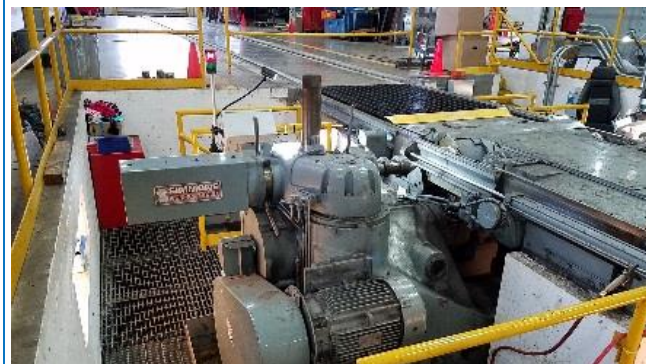
Wheel Truing Machine (Below Grade), Orient Heights Maintenance and Storage Facility
