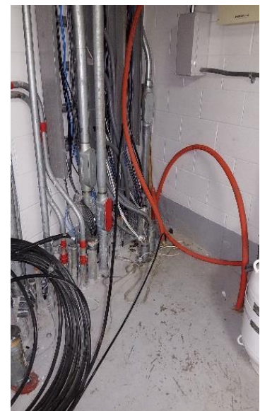
Communications Cables, Airport Station
