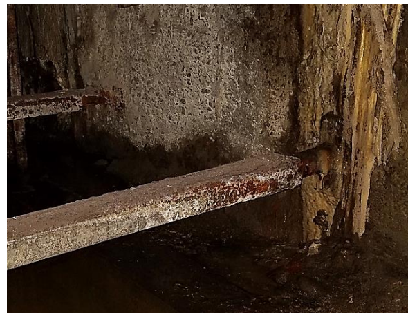
Exhibit 7. Visible Evidence of Exposure to Saltwater at Aquarium Station.
