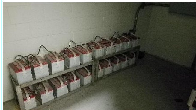
Emergency Battery System Packs, Wood Island Station
