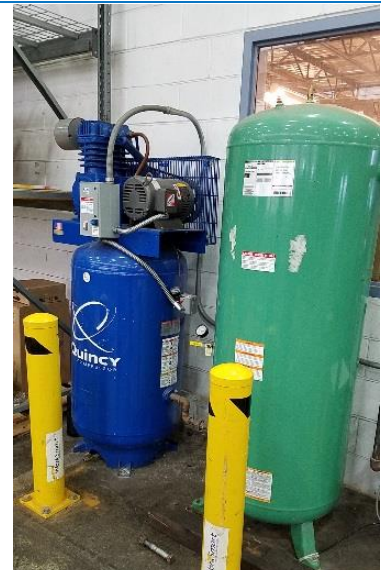
Hydraulics Equipment, Orient Heights Maintenance and Storage Facility
