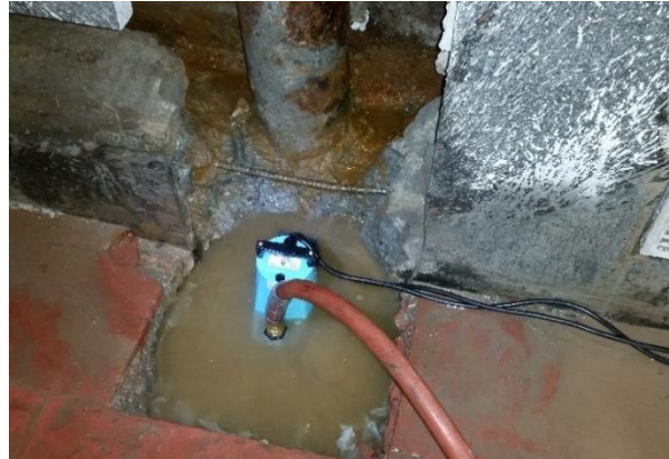
Exhibit 8. Drainage Trough and Pump at Aquarium Station
