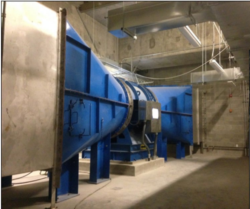
Figure 15-2. A Single Tunnel Ventilation Fan Installation of Similar Type, Size and Arrangement
